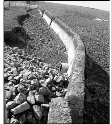
The Lowman Beach Park seawall has cracked and shifted to the point that it is allowing erosion. Photo courtesy Seattle
