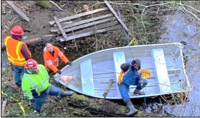
Removing the partial culvert blockage under 45th Ave. SW required a lot of hard labor and, yes, a boat to navigate in "Fauntleroy Pond." Photos courtesy Tom Trulin
